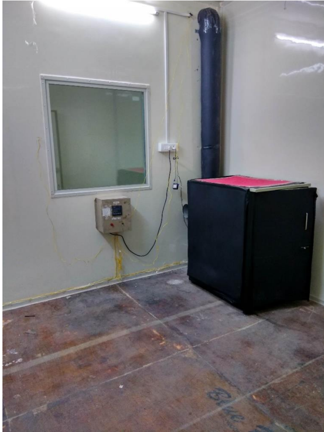
Heat exchanger set up in the room
